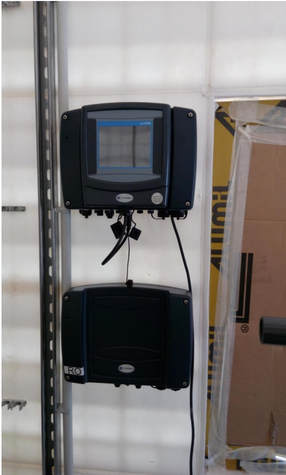
Figure 12: MBR –RO instrument controllers
