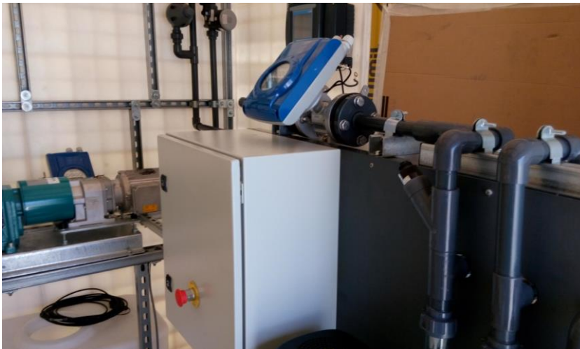
Figure 13: RO MCC panel
