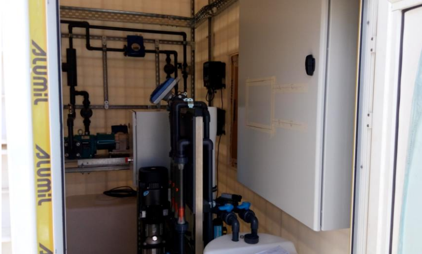
Figure 14: MBR MCC panel
